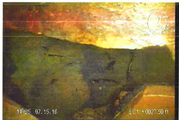
#6: Pipe Defect at 27.5 feet from MH 6-025 (tap break-in, hole void visible)
