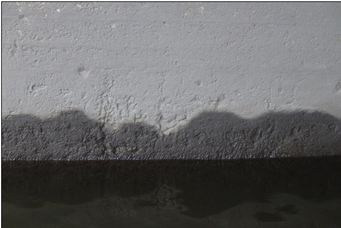
Photograph 12: View of Concrete Scaling at the Waterline at the Downstream Quarter-Point on the East Face of the West Pier, Looking West.
