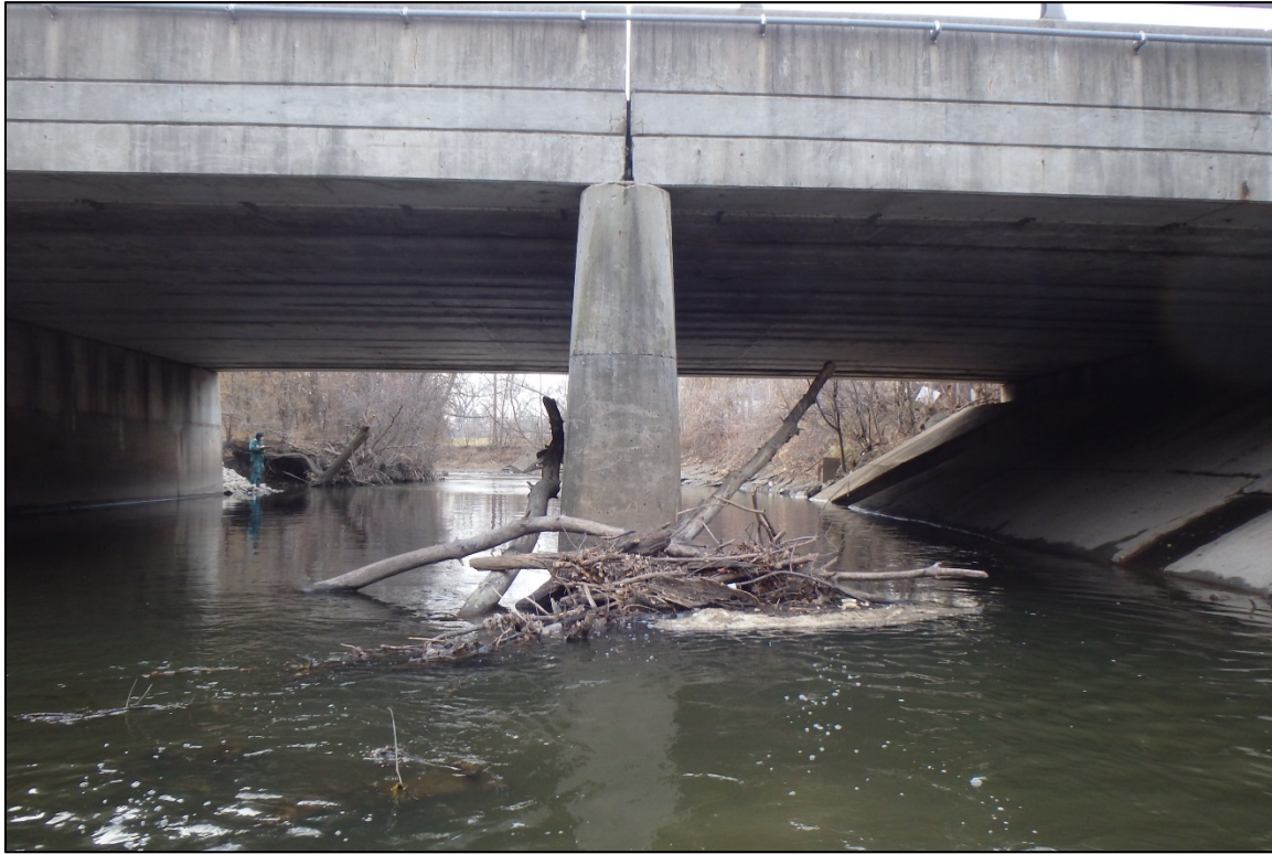
Photograph 15: View of Timber Debris Accumulation at the Upstream Nose of the West Pier, Looking South.
