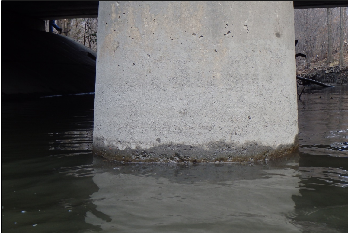
Photograph 11: View of the Typical Concrete Condition at the Waterline at the Downstream Nose of the West Pier, Looking North.
