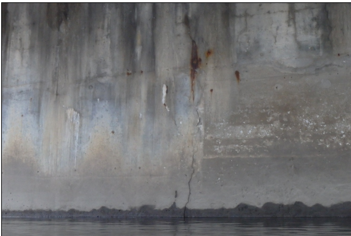
Photograph 18: View of a Typical Crack in Construction Joint on the West Face of the East Pier, Looking East.
