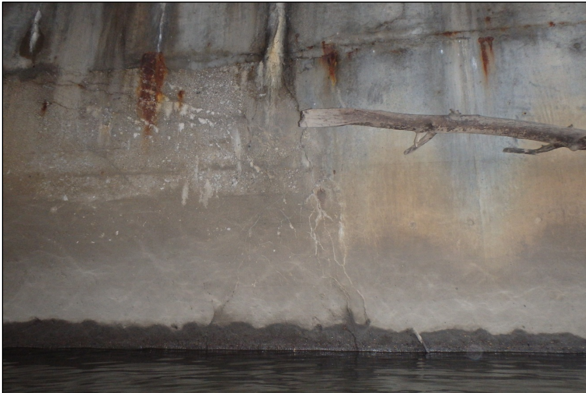
Photograph 13: View of Cracking at the Upstream Quarter-Point on the East Face of the West Pier, Looking West.
